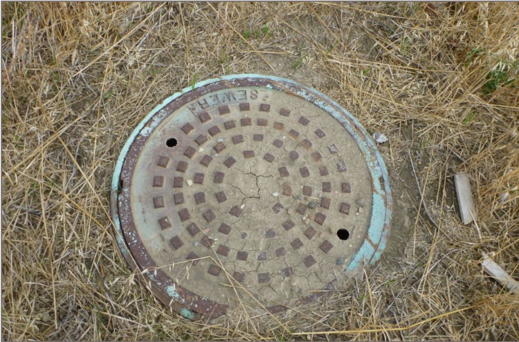
Photo 3: Sanitary Sewer 2 found within Suspected Wetland 1.
