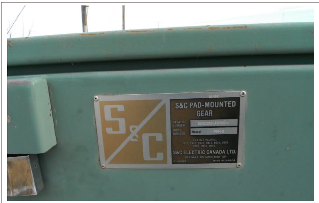
Photo 10: Transformer located on the northwest side of the site.
